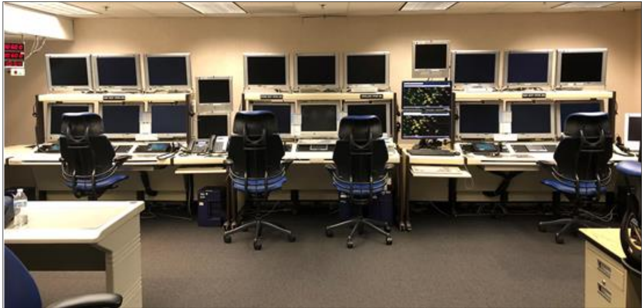
Figure 6.2-2. Range Safety Room Console
