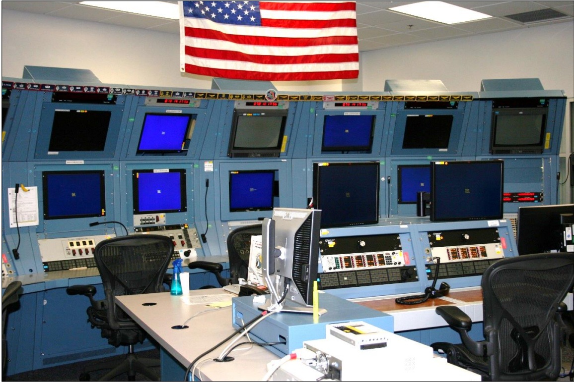
Figure 7.3-3. CCAFS Safety Control Room
