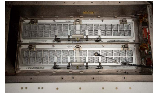
Siloxane Filters Installed on ISS
