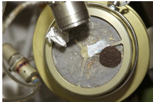
Inlet to avionics cooling fan
