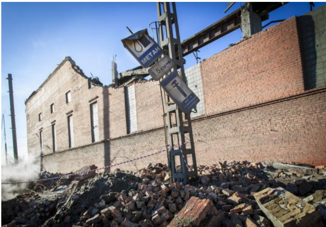
Figure 35. Damage to the zinc plant in the city of Chelyabinsk. Image credit: Oleg Kargopolov/AFP/Getty Images.
