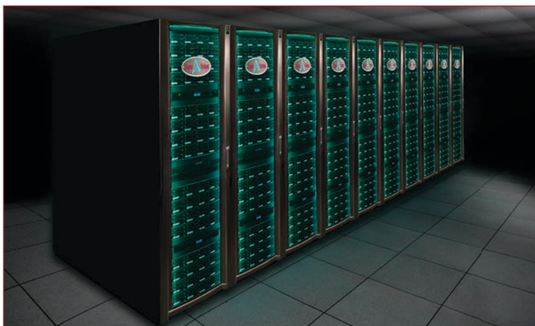
Scalable Compute Unit 15 (SCU15) is part of the Discover supercomputer cluster at the NASA Center for Climate Simulation (NCCS). SCU15 was installed in July 2019. It is an expansion to the Skylake and Omni-Path portion of the Discover cluster. Chris Meaney, NASA/Goddard
