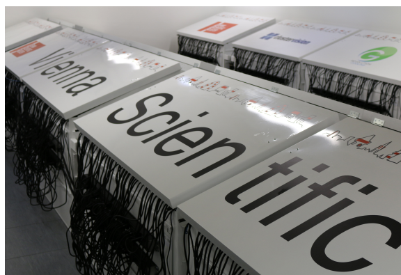
Fig. 1 Picture of the room where the 2020 nodes with liquid submersion cooling of the VSC-3 are stored. Picture was taken at VSC Arsenal TU Wien building ©Claudia Blaas-Schenner.
