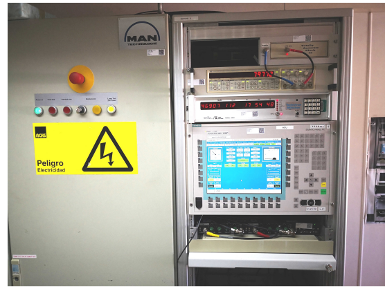
Fig. 5 Servo cabinet with antenna control unit inside the AGGO-2 VLBI operation container.
