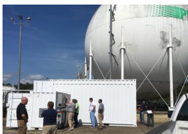
Figure 23. Helium Recovery System (HRS) being readied for commissioning at NASA Stennis Space Center.
