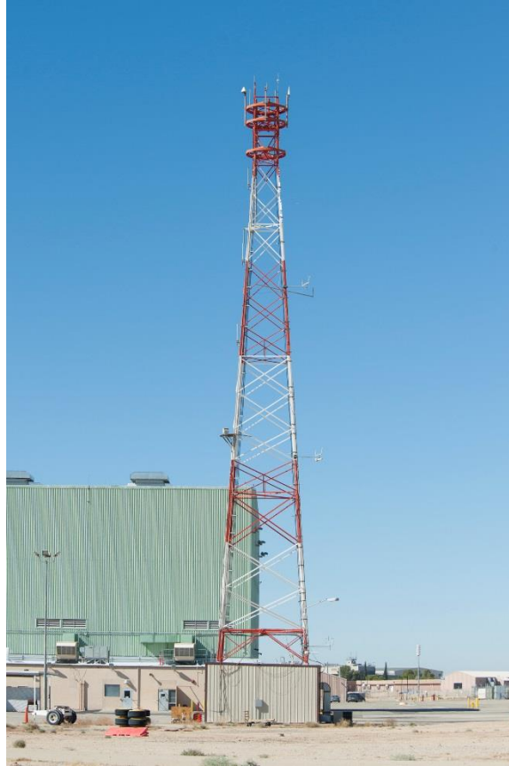
Figure 45. Tower used for mounting ultrasonic anemometer near primary array for AFRC test.
