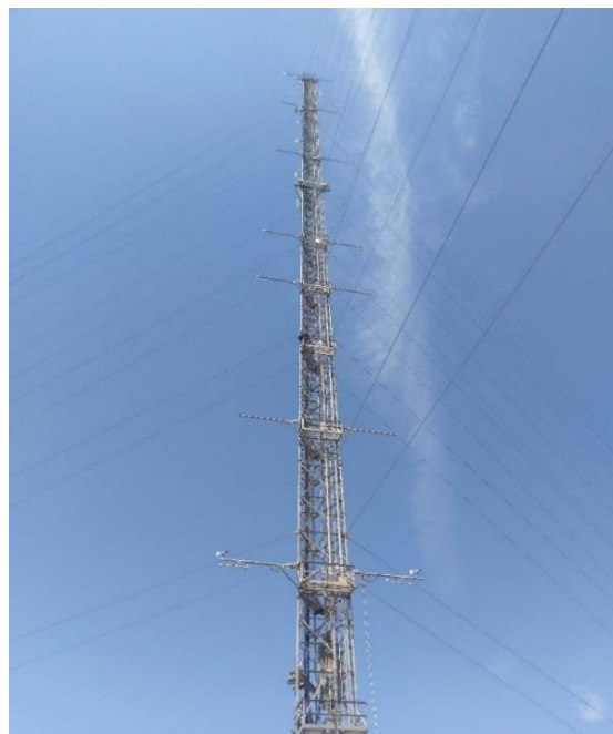
Figure 96. 150 meter tower and mounting arms.
