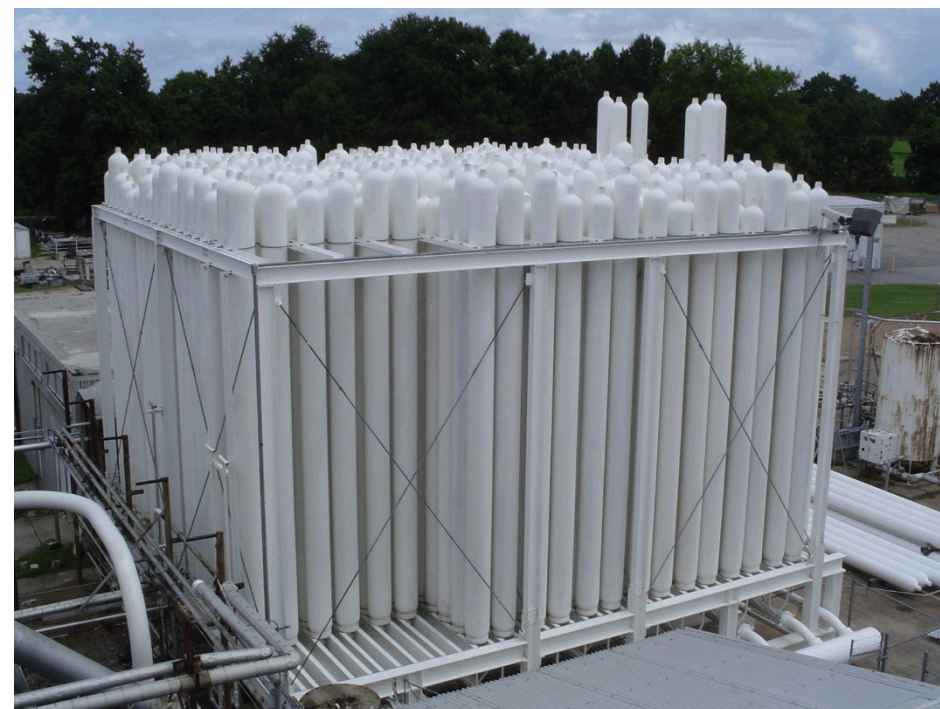
8' HTT - Compressed air storage
