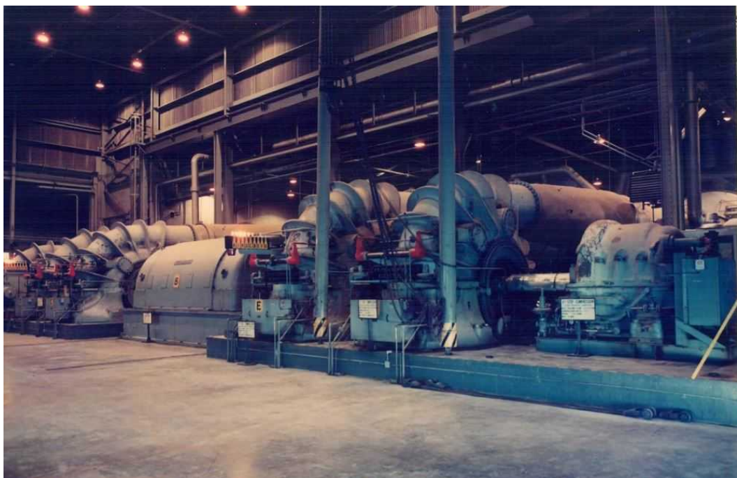
UPWT drive line - compressors
