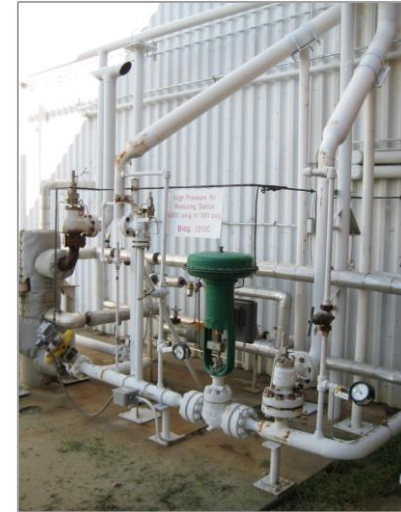
Air Reducing Station
