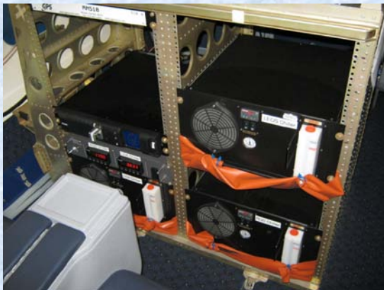
Three laser chillers
