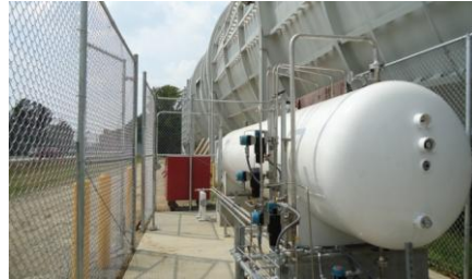
Propane Fuel System
