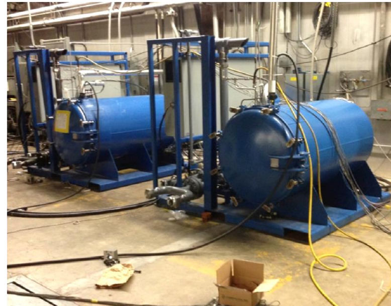
Two portable valve pallets underneath wind tunnel control propane delivery to CJES units
