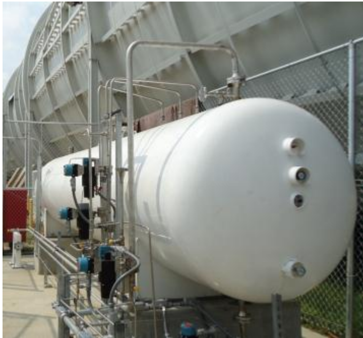
2500 gallon liquid propane storage tank
