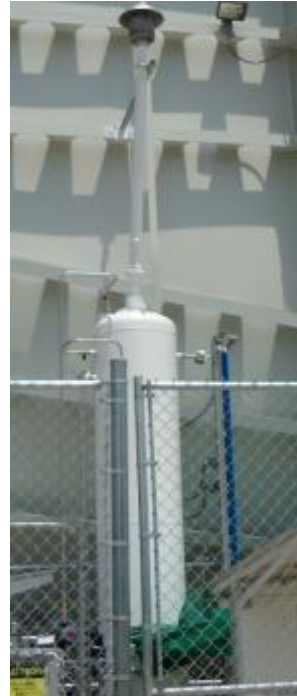
500 gallon run tank
