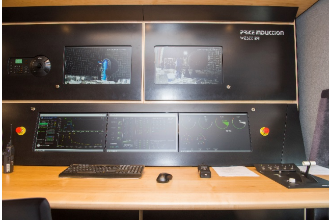
Akira Mecaturbines Control Station
