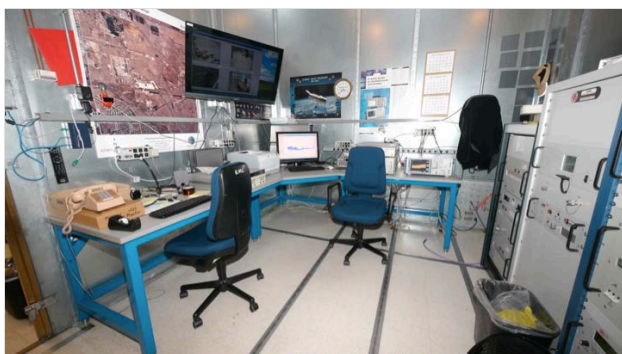
Figure 18. Large EMC Control Console
