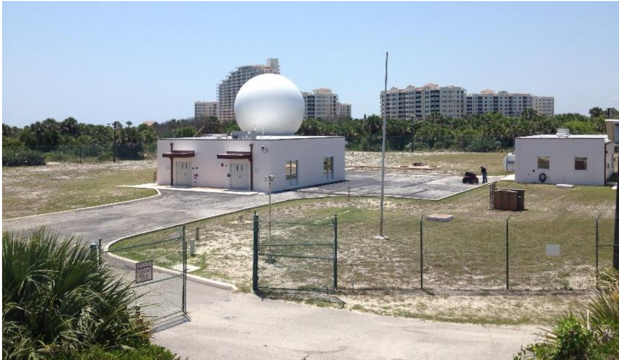
Figure 8-2. PDL Ground Station
