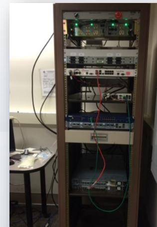
Testbed Network Equipment
