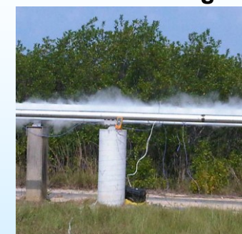
Cryogenic Fuel Line Monitoring
