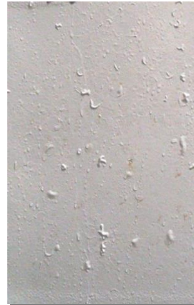
Blistering of Acrylic Topcoat over Inorganic Zinc
