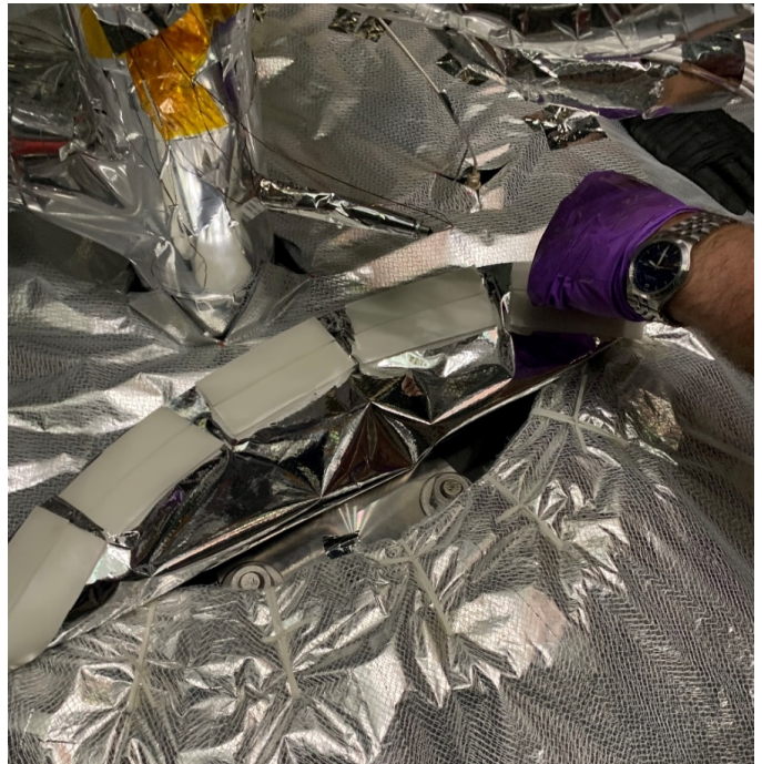
Figure J.18.—Attaching manway cover onto the first subblanket on the forward dome.
