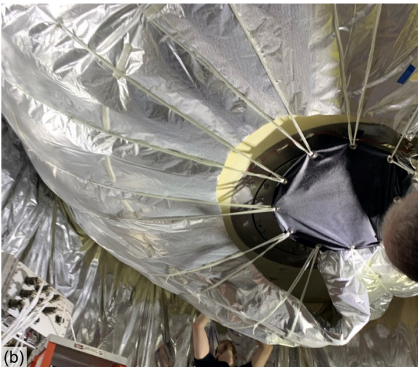
Figure J.12.—Installation of the first subblanket on the aft dome. (a) Beginning installation. (b) Installation almost complete.
