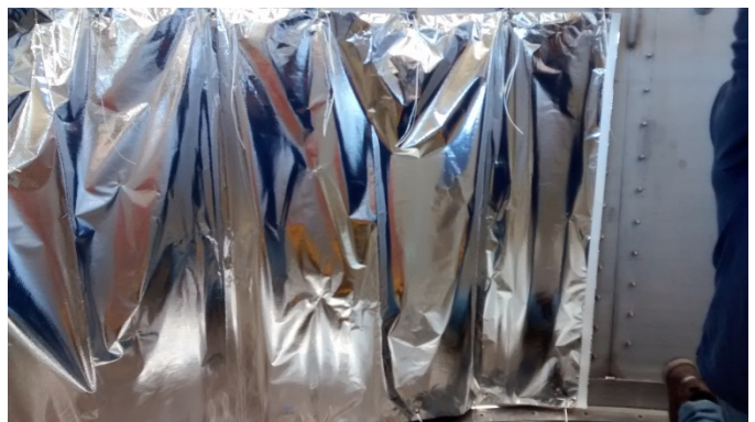
Figure J.9.—Multilayer insulation being installed on the inside of the aft skirt.
