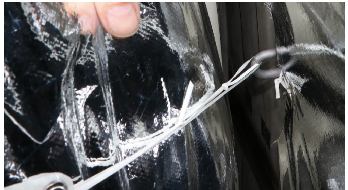
Figure J.19.—Closeup image of lacing cord attachment from structural patch to tiedown and gap area above multilayer insulation blankets in Y-joint of the aft dome and skirt.
