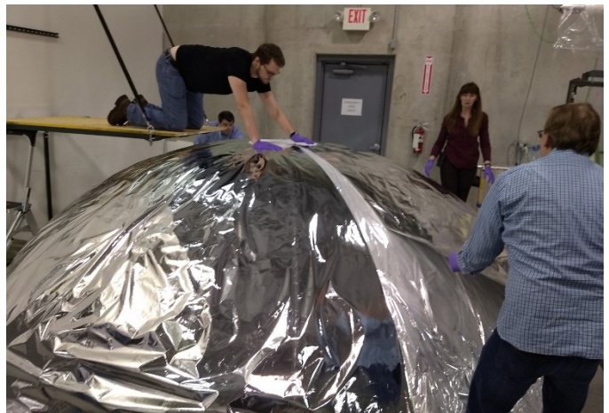
Figure J.8.—Installing multilayer insulation layers on the Structural Heat Intercept, Insulation, and Vibration Evaluation Rig (SHIIVER) dome mold.
