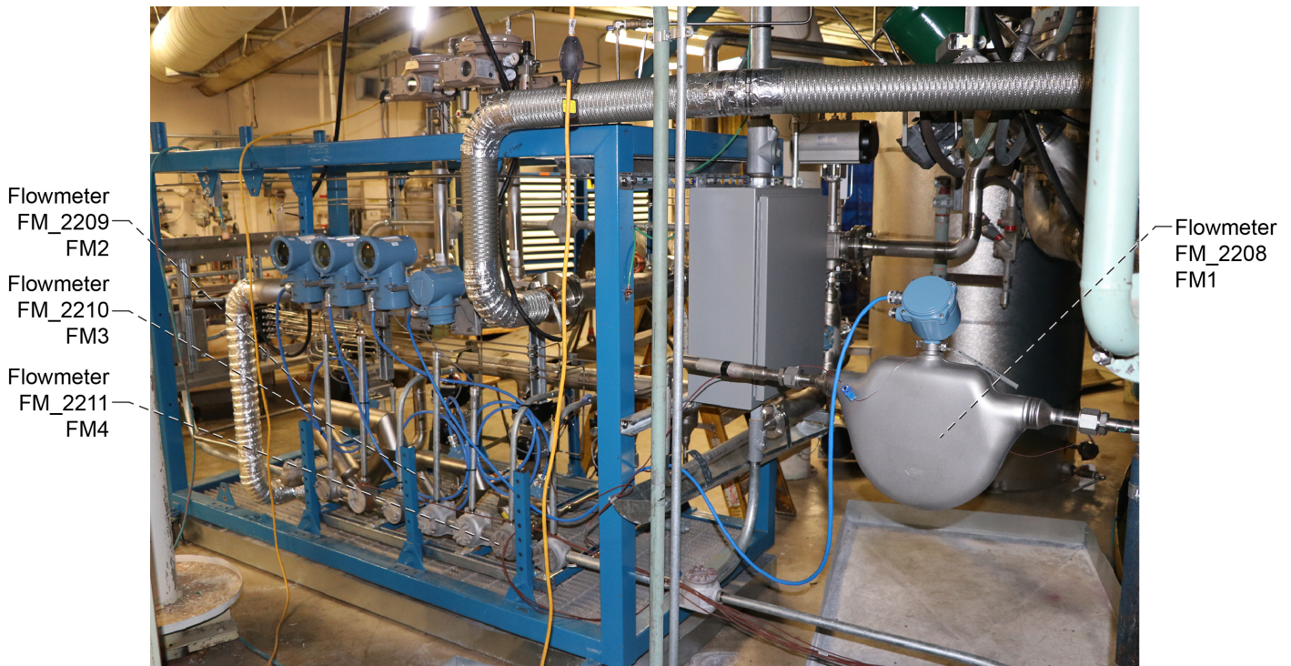
Figure 24.—Backpressure control cart.
