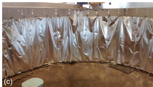
Figure 13.—Installation of multilayer insulation. (a) Dome mold. (b) Interior of forward skirt. (c) Aft skirt.
