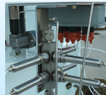
Sensor probe assemblies mounted in a flow-through manifold
