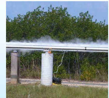
Cryogenic Fuel Line Monitoring
