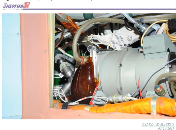
Figure 4. Photograph of Pretreated Urine Leak from Urine Separator
