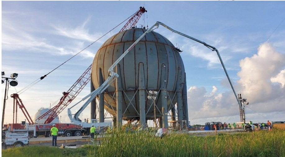
Figure 8. New 4,700 m 3 LH 2 tank under construction with prior 3,200 m 3 tank in background.
