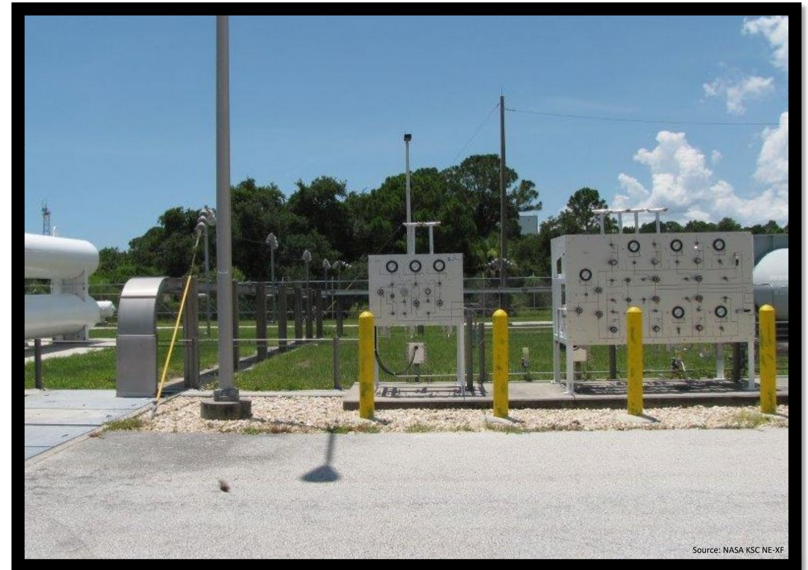
Figure 4. MPPF Facility Pneumatics System
