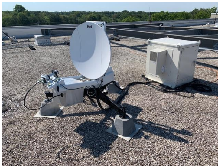
Preparing for testing with O3b – APL rooftop
