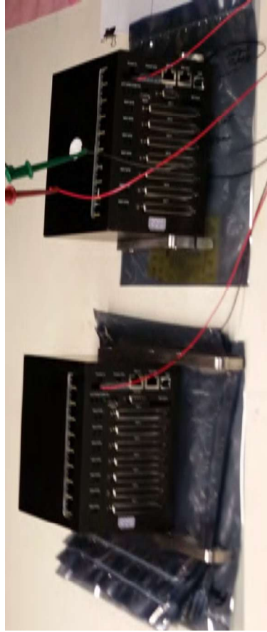
UEI Data Cubes (Thermocouple Signal Conditioning)
