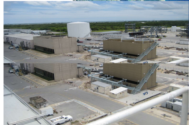
Industrial Area Chiller Plant
