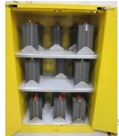
Battery System Ship Set (16 modules)
