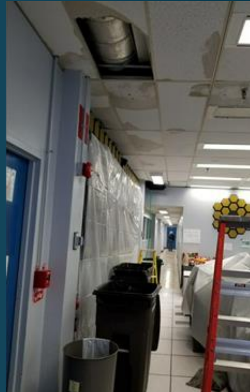
Water Damage in OTIS CV Test Control Room Source: NASA/L. Feinberg
