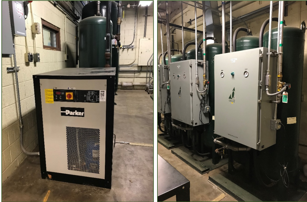
Figure 3.—Left: Refrigerated air dryer and the service air receiving tank holding the dried air. Right: Bank of three OG-500 oxygen generators.
