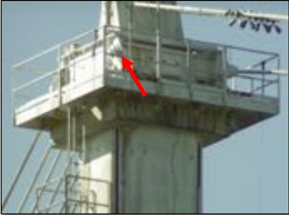
Tower 4 w/ M4N Socket
