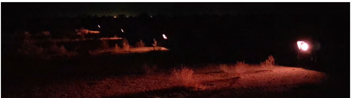
Figure 12: Four PAPI lights with red beam visible at night on the ground.
