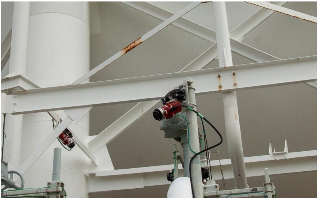
Figure 3: Launch complex 39-B (LC-39B) hydrogen facility as recently modified after the Space Shuttle program for the Space Launch System. Shown on close-up (bottom image) is one of the new model fire detectors, a Det-Tronics infra-red flame detector focused on water-band emissions. Ultra-violet detectors by the same company have also been installed.
