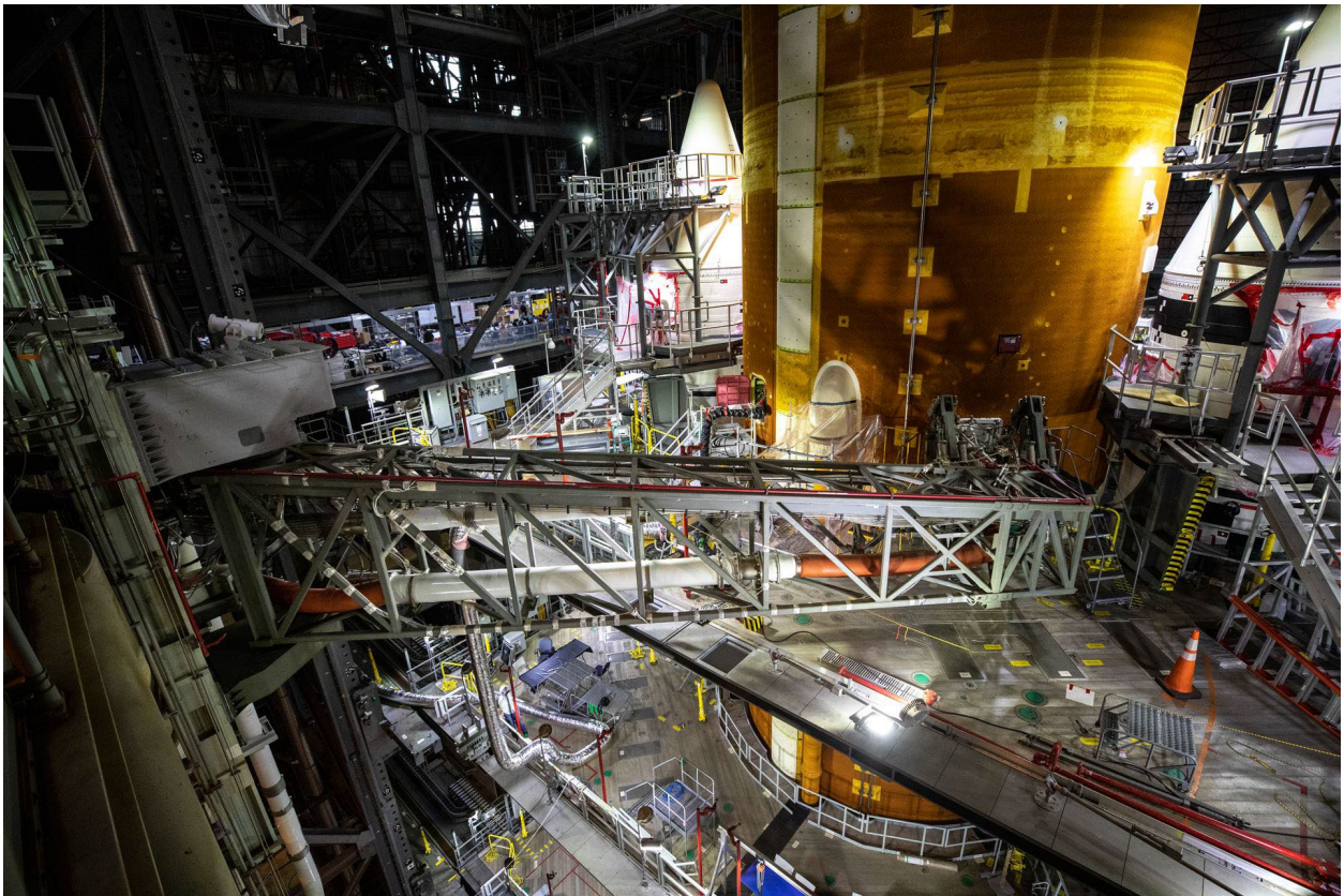
Figure 7: The core stage intertank umbilical – one of multiple connections on the mobile launcher that will provide power, communications, and pressurized gases to the rocket – is attached to SLS in the VAB as part of the ITCO test series.
