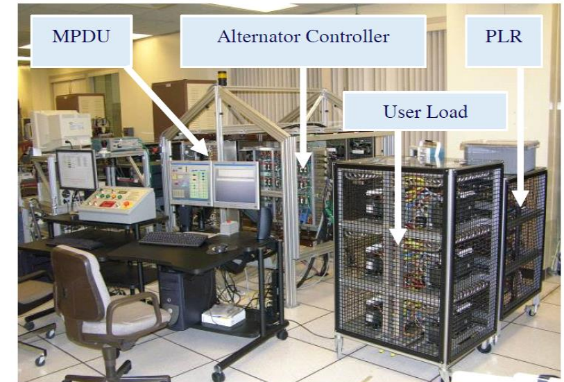
Lunar Power System Facility at GRC
