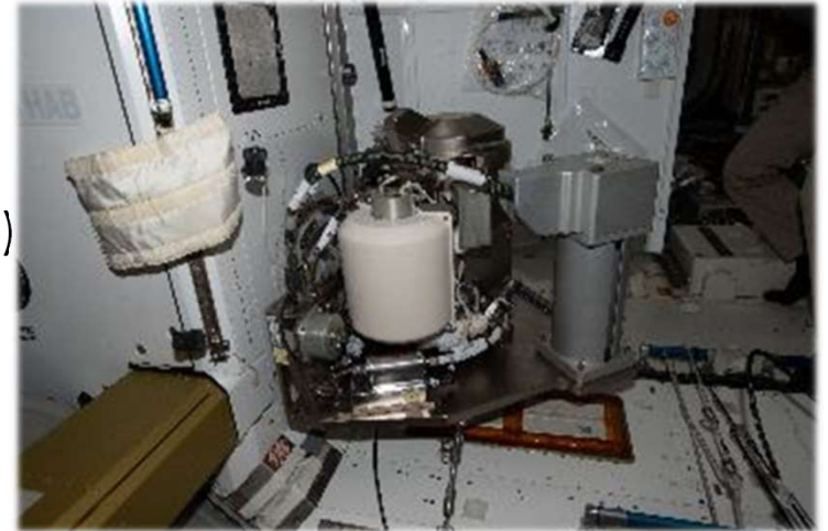
ISS UWMS installed in Node 3, ISS
