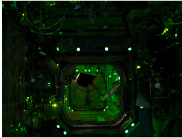
Figure 90: An example of photoluminescent dots used for emergency egress lighting on board the ISS.
