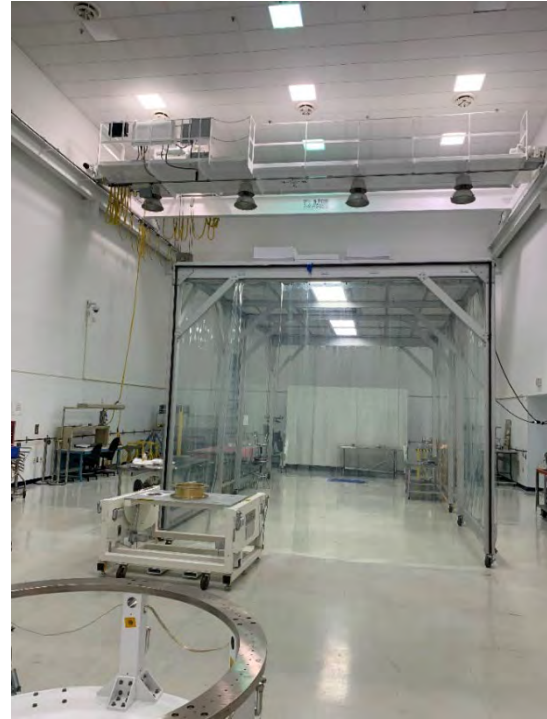
Figure 58: High Bay East Cleanroom Tent with ESPA ring integration ground support equipment in the foreground
