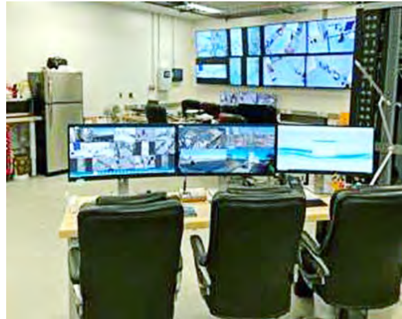
Figure 82: MARS Payload Processing Facility Control Systems
