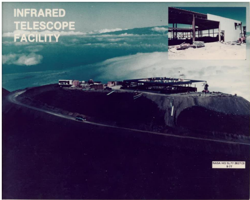
Figure 1 Aerial photo of construction of the NASA Infrared Telescope Facility. Photo credit: NASA HQ Archives.
