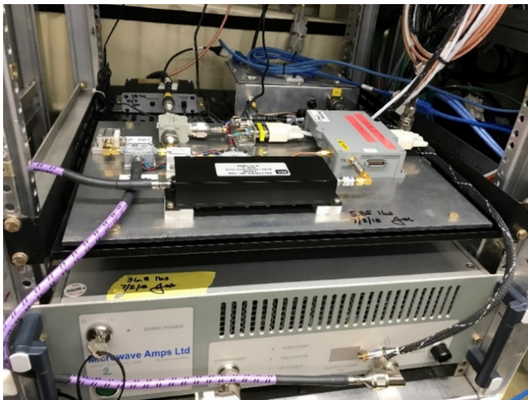
Figure 9.—CNPC-5000E radio on transmit and receive plate with high-power amplifier below.
