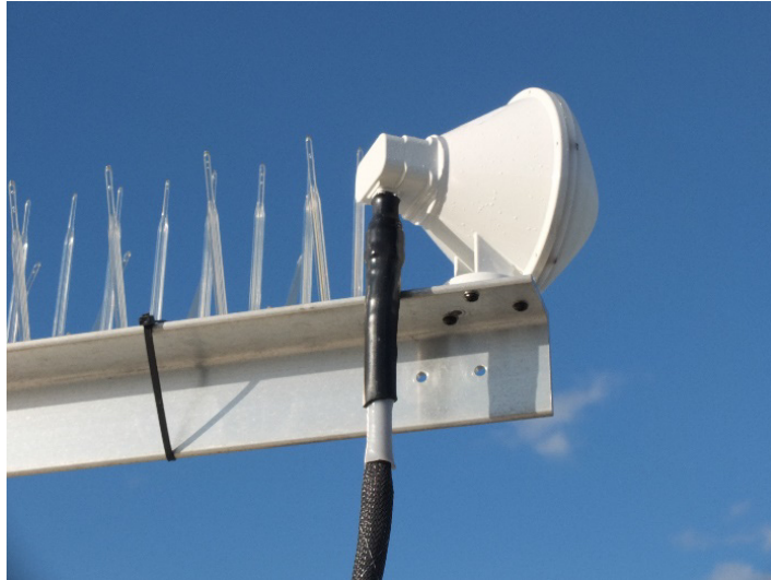
Figure 20.—Installed ground station directional antenna.
