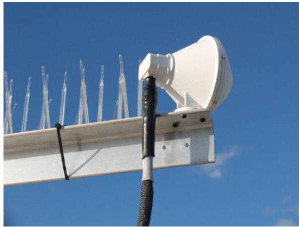
Figure 8.—Installed ground station directional antenna.
