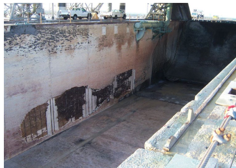
Launch Pad Flame Trench Damage
