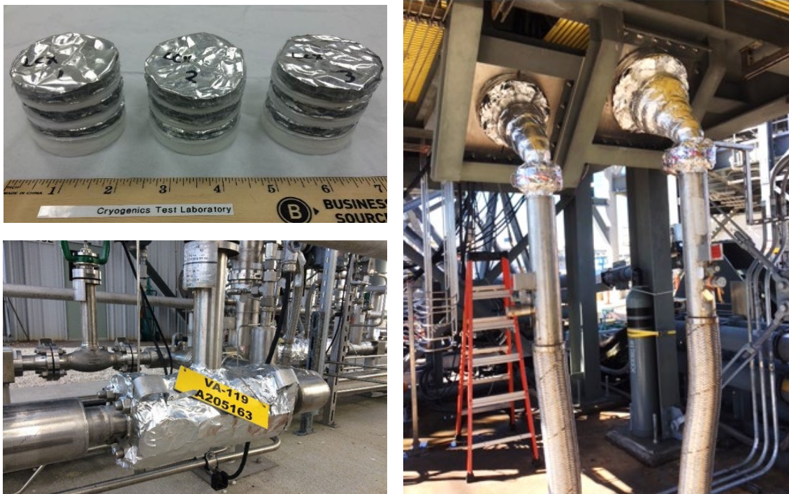
Figure 5. LCX Sample Stack-Ups with Three Layers of Aerogel Blanket (upper left); LCX Insulated LH 2 Valve (foreground) and Uninsulated Unit (background) (lower left); LCX Installed on LH 2 Fill & Drain Ports (right)
