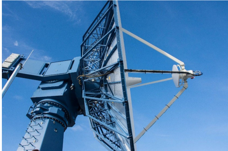
Figure 11.12: Ground Antenna in Fairbanks, Alaska. Credit: NASA/ Clare Skelly.
