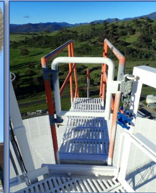
New Access Gate at Apex
