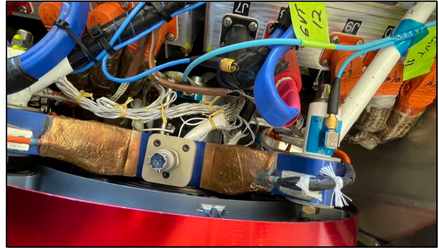
Close quarters in the nacelle resulted in unintentional grounding
