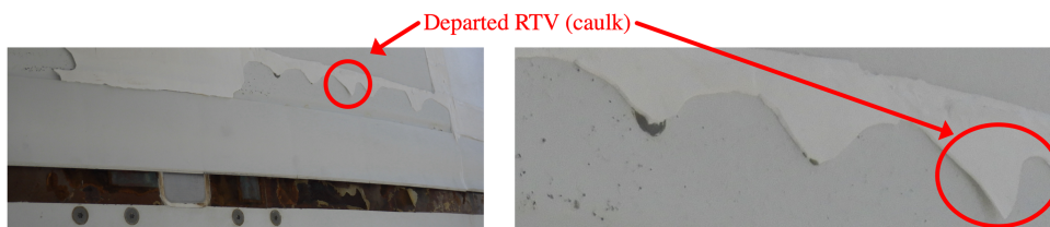
Fig. 21 Images of RTV damage to SLS resulting from Hurricane Nicole. (Photographs: NASA)
