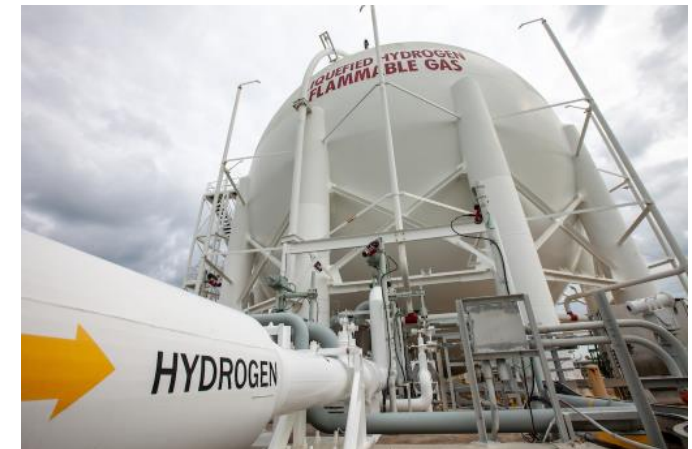
LH2 Storage Tank and transfer line at NASA KSC
