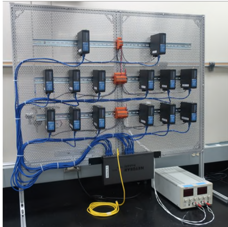
Figure 10. Control system hardware/ software demonstrator
