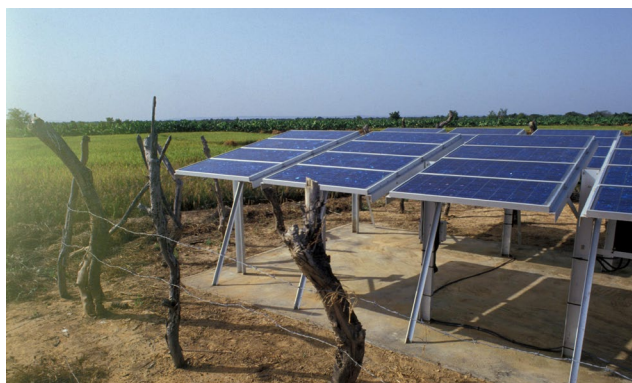
Solar panels on a farm Mali Photo © Curt Carnemark World Bank.jpg
